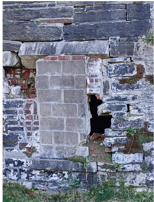
Fort Ives Wall - Granite Transom Door Collapse Oct 2024 Photo credit: Cathy McCarthy
