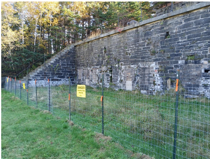
Fence blocking access to Fort Ives Wall Photo Credit: Cathy McCarthy
